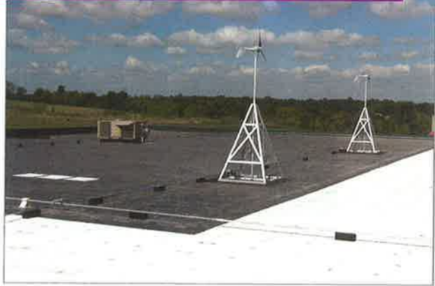
An infrared scan shows the lower temperature of the coated portion of this EPDM roof.
