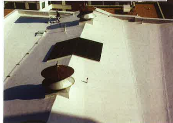
A 14-year-old built-up roof system before and after coating. The roof, coated in 1996, was recoated within the next five years to extend the coating's life.
